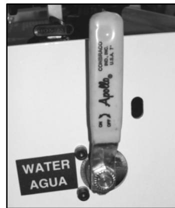
Figure 17: Water Valve Assembly
